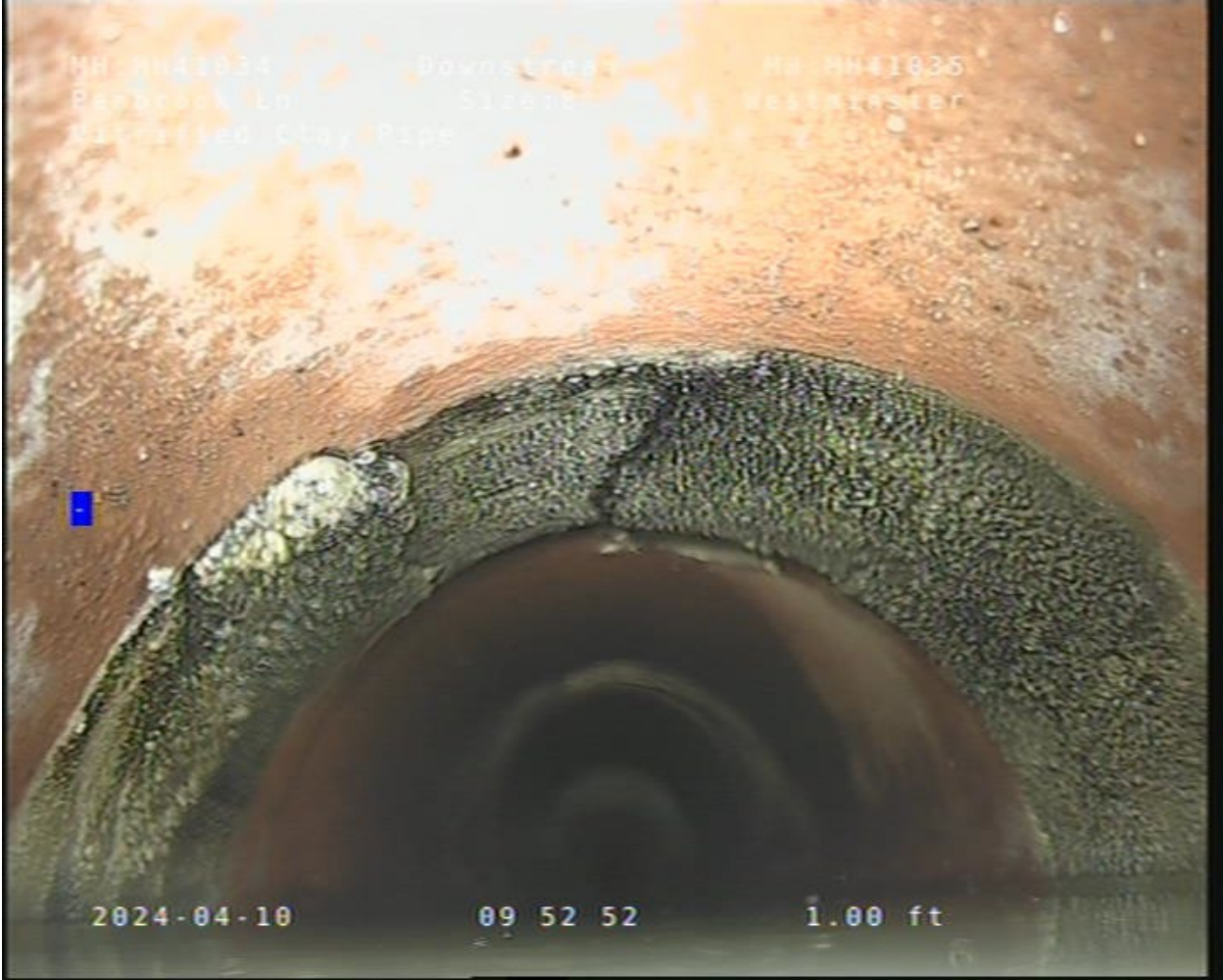
Photo #2 - 04/10/2024 – CCTV photo of a damaged pipe a few feet east of manhole number 2006
