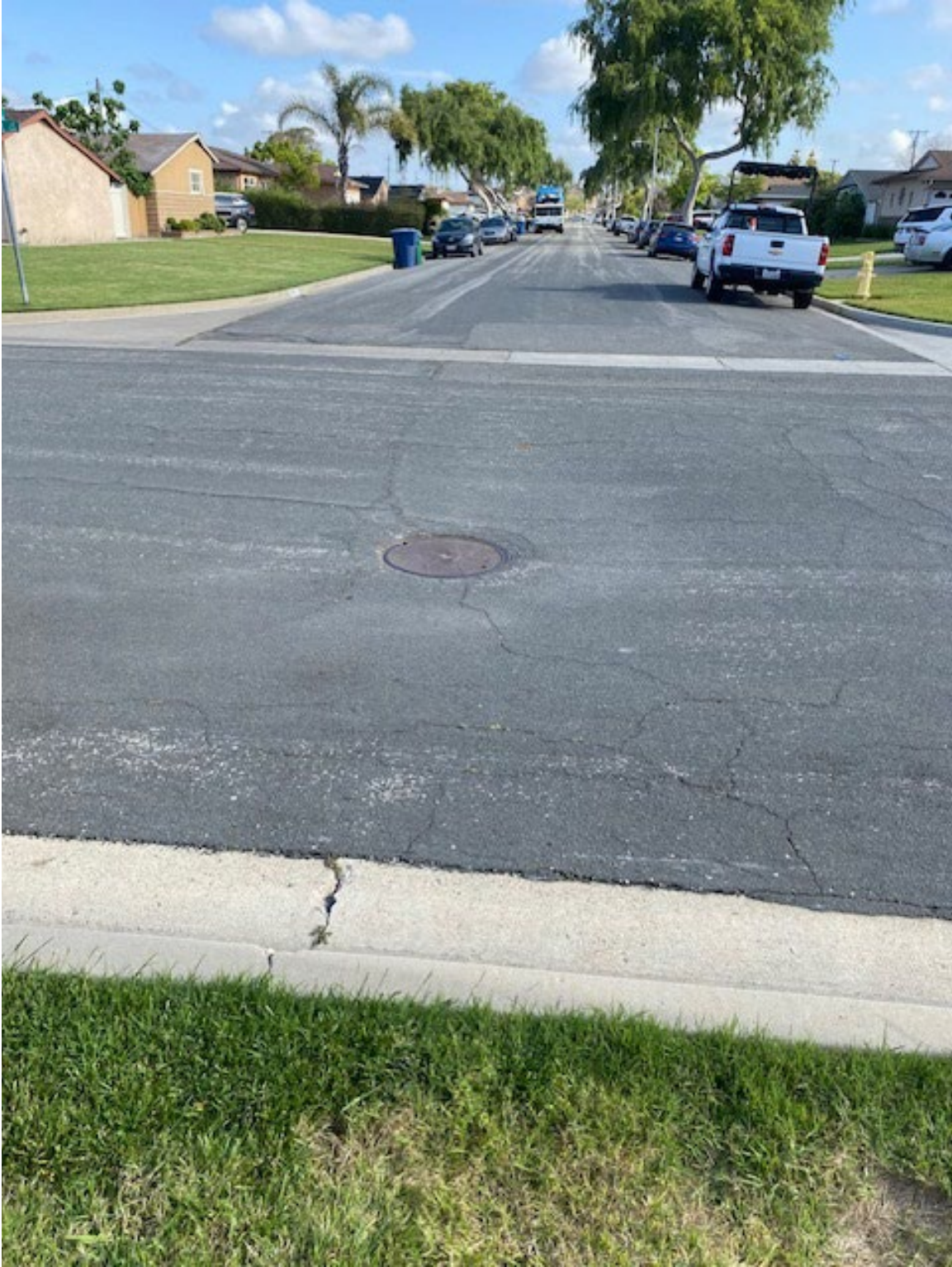
Photo #3 - 04/24/2024 – subsidence street and subsidence manhole number 2006 at the intersection of Pembroke Lane and Webber Place (looking north)
