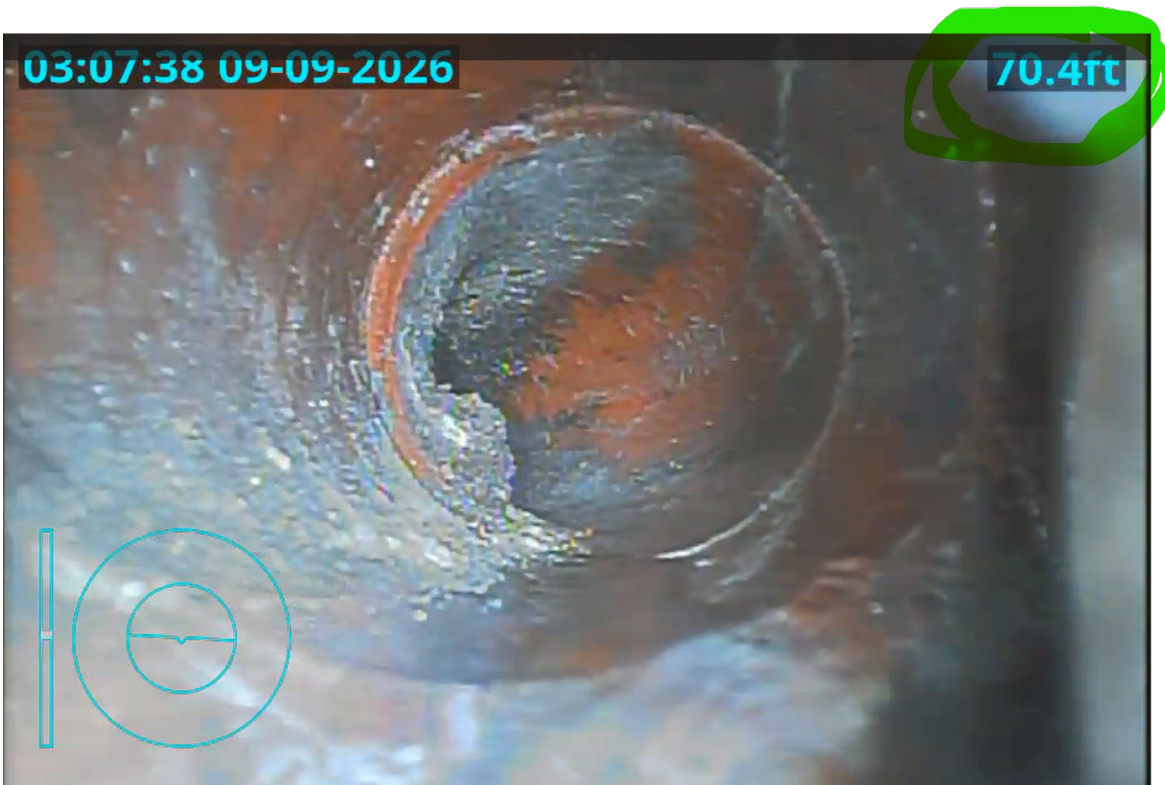
Proposed camera system. First lateral on Moran St. Properly working footage counter.
