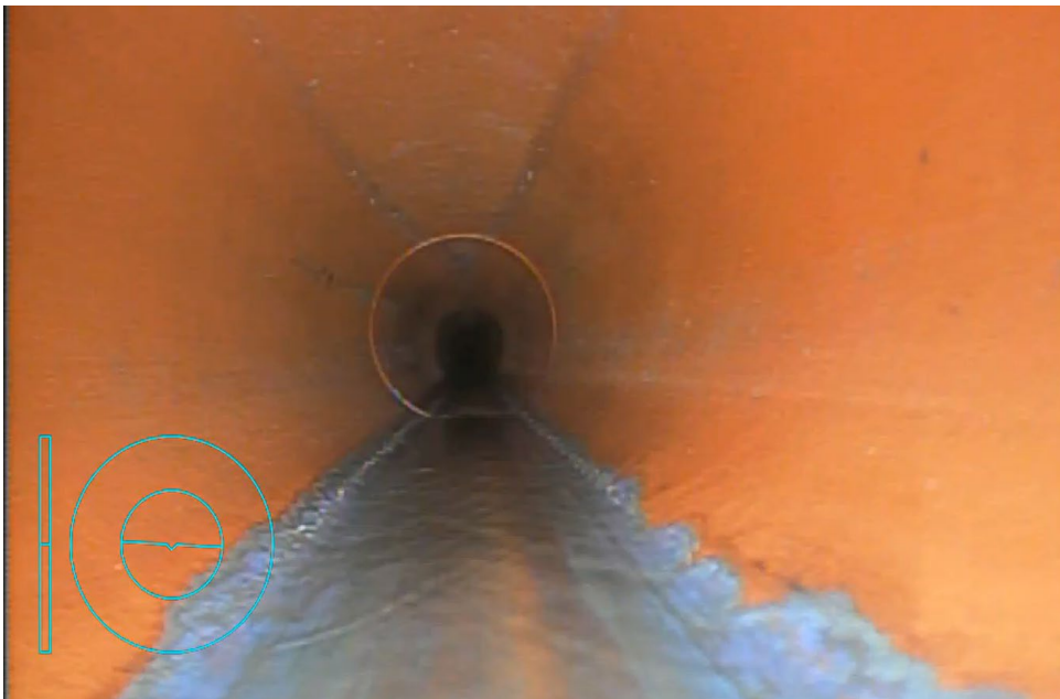
Proposed camera system. Beginning of Moran St. pipe segment.
